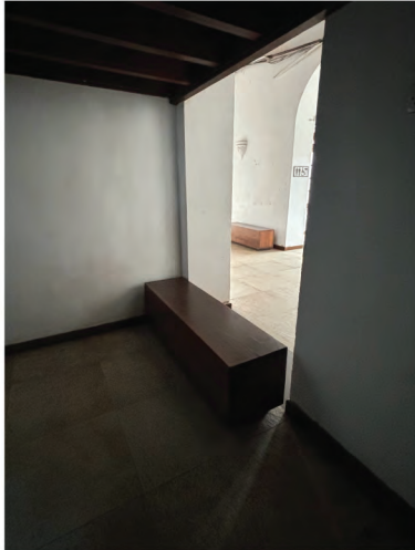
Figure 15 : Corridor blocked off
